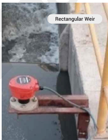
Effluent Treatment Plant
