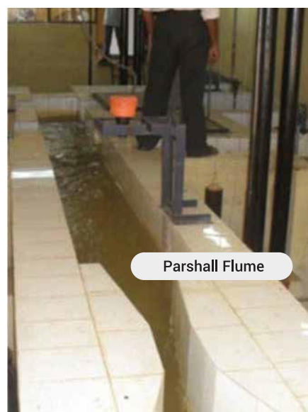
Sewage Treatment Plant
